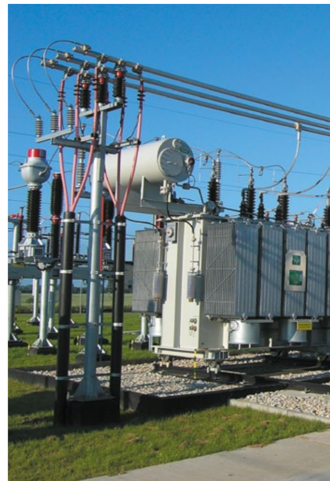
Transformatory o mocy 31,5 MVA i 25 MVA, Elektrownia Wiatrowa Tymień Transformers with rated power of 31,5 MVA and 25 MVA, Windmill Power Plant Tymień
